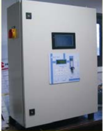
O 2 -CO 2 automatic controller
